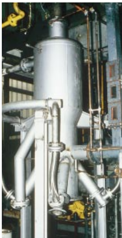
Figure 1: Pyrolysis reactor capacity 20kg/h small pilot plant.
