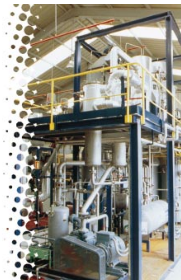
Figure 1: Pilot plant of 200kg/h of dry biomass. Meirama, Galicia (Spain).
